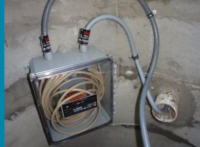
AFO Cable splice point
