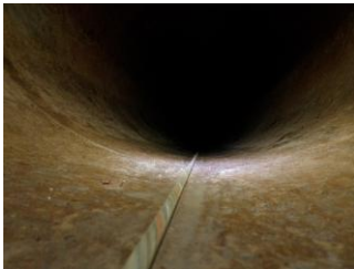
AFO cable in pipe
