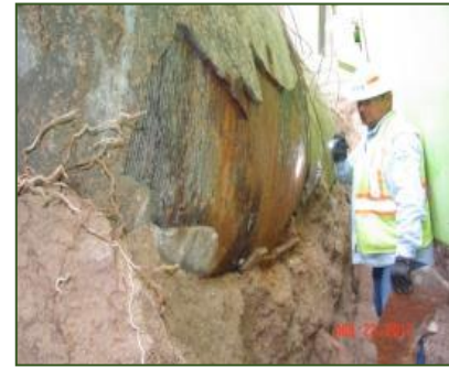
Inspecting the damage
