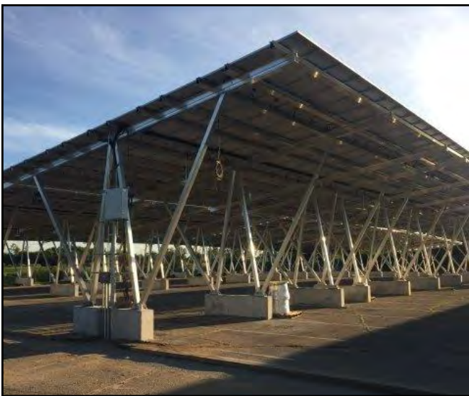
Figure D18: Solar arrays built in parking lots on Michigan State University's campus
