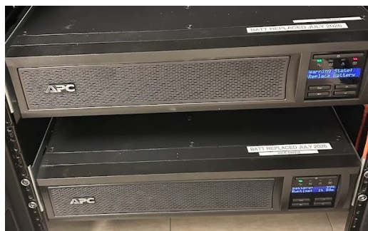
Rack-mounted UPS with fresh new batteries installed by Denise and Jeff
