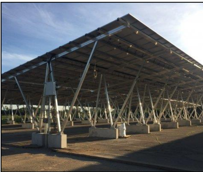
Figure D15: solar arrays built in parking lots on Michigan State University's campus
