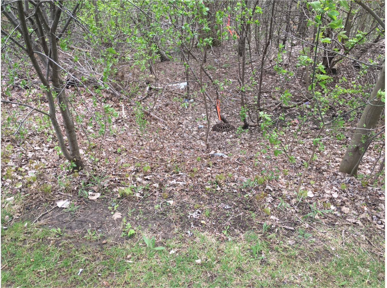
Site Photograph: Low depression area and yard basin on Saddle Creek property, north of Woodbridge Lane
