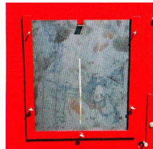
K-12 plunge cut window for hooking & releasing panic bar with framing square.
