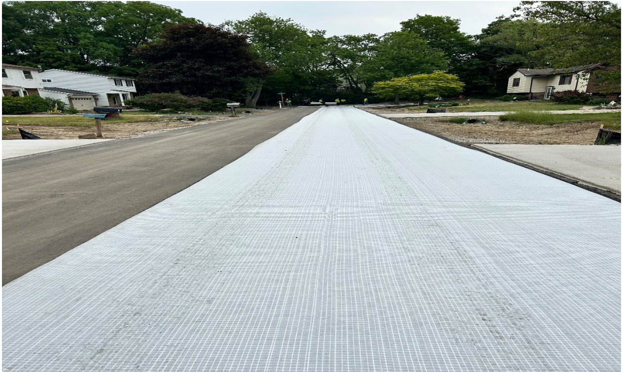
(After) Wainwright Street – Looking east from Martin Avenue – Placement of Interlayer Fabric
