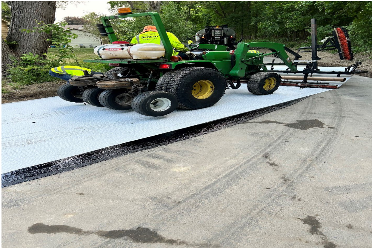
(After) Paramount Street at Linhart – Placement of Interlayer fabric before final asphalt wearing course
