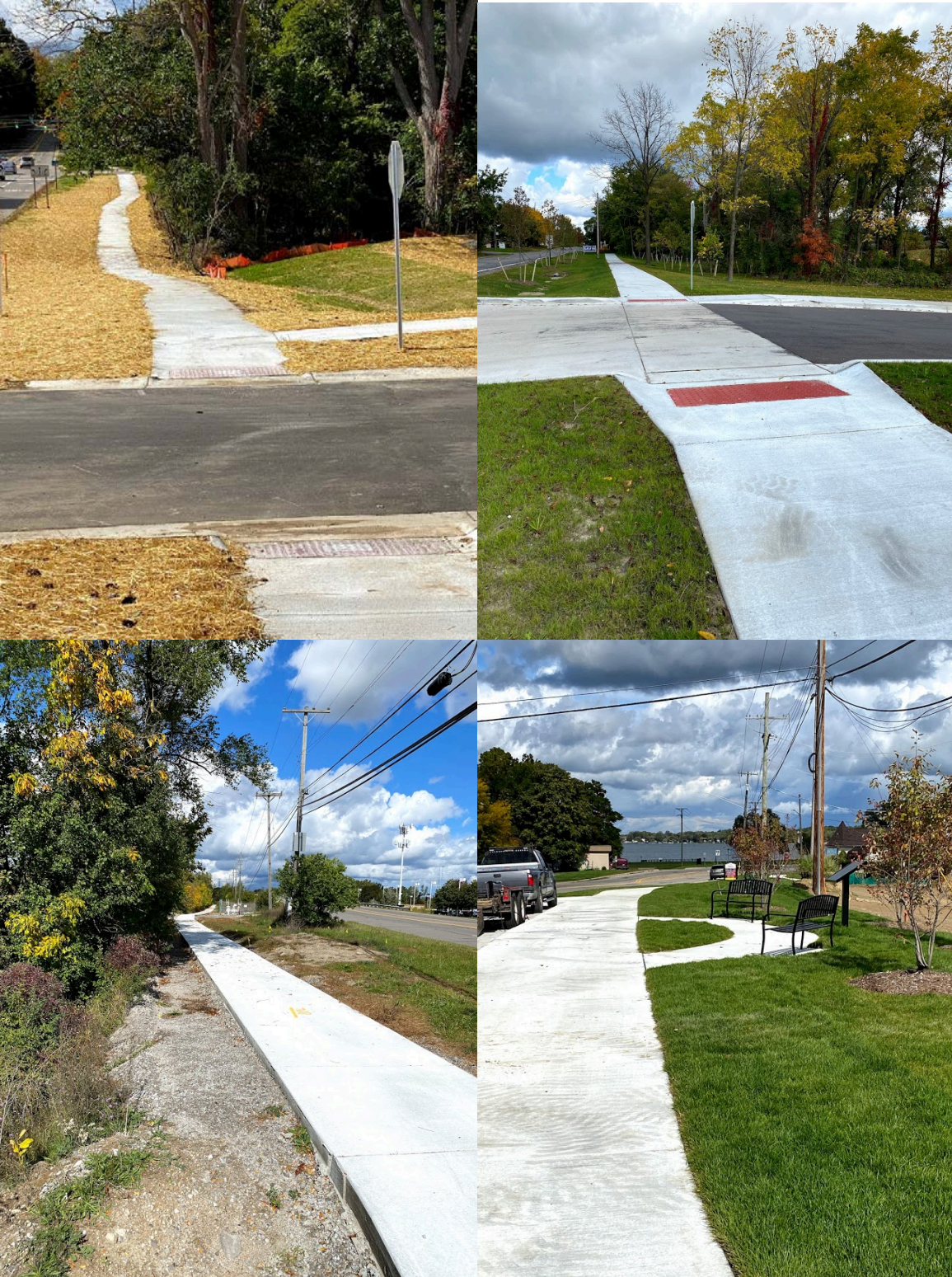
Private development contributed to new sidewalk segments along Nine Mile, Seeley Road, Haggerty Road and Old Novi Road
