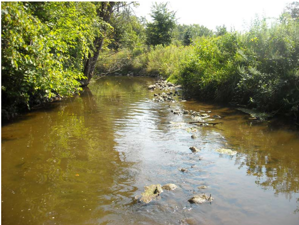
Riprap in channel showing pre-erosion bank location (looking downstream)
