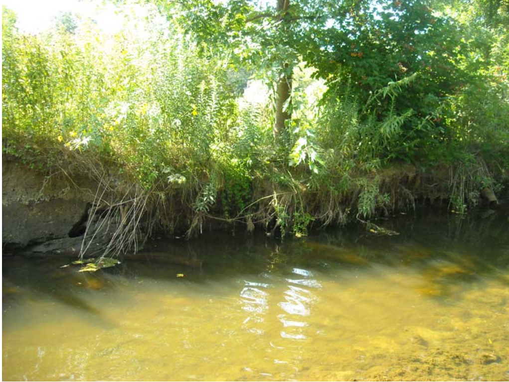
Outside Meander Erosion & Undercutting Bank, Bank Height = ~ 3.5', BEHI =31/Very High
