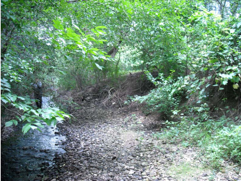
Upper Bank Slope Failure, looking downstream, Bank Height = ~ 5.5', BEHI = 31/Very High
