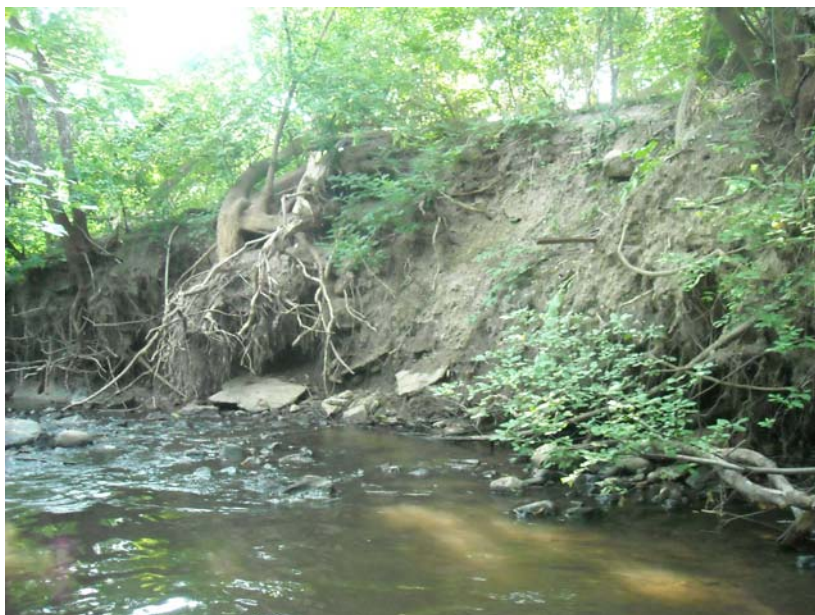
Active Bank Erosion at downstream end of Site 7
