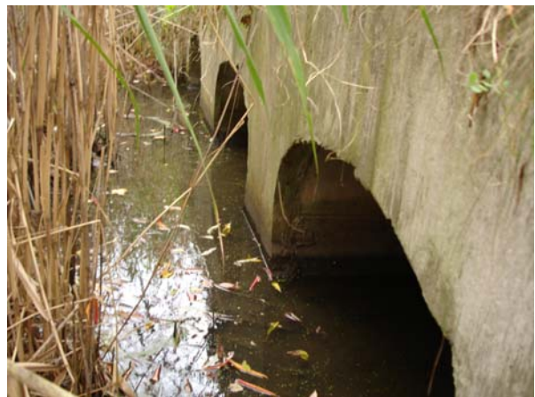
Novi Road Crossing
