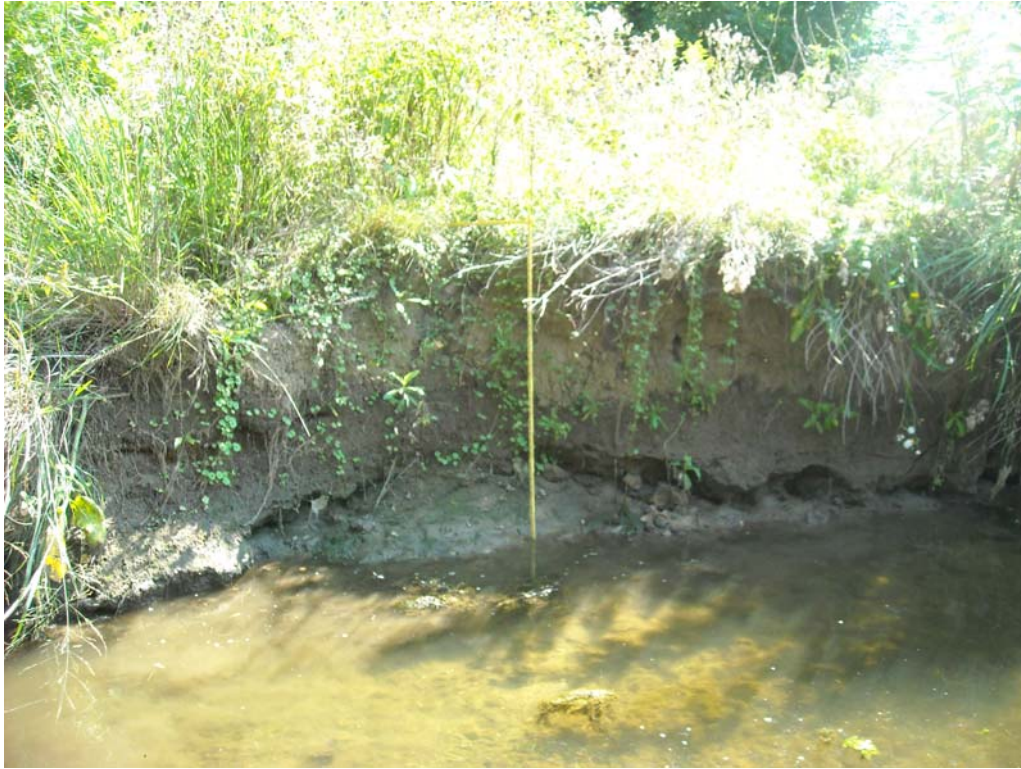
Active Bank Failure and Slumping
