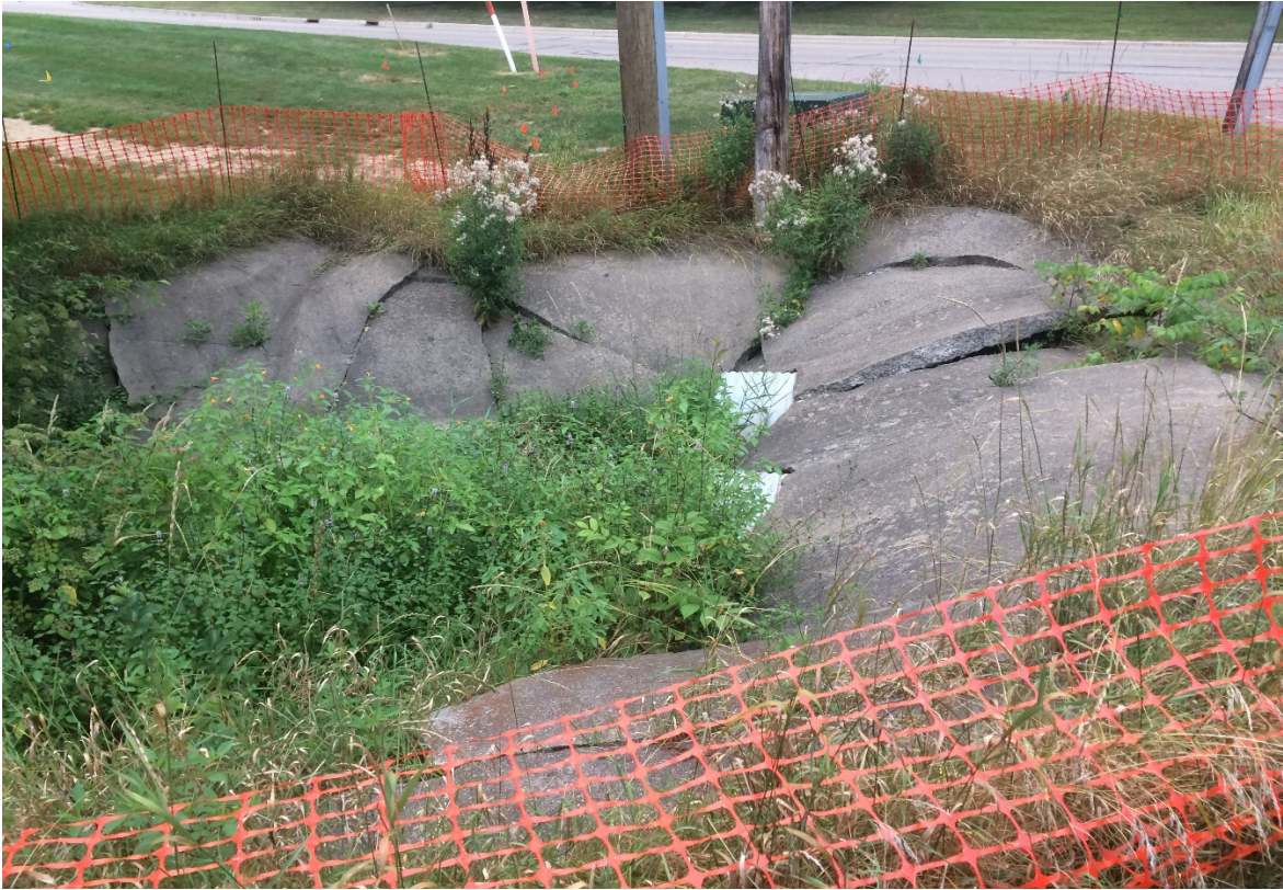
Thornton Creek culvert crossing at 9 Mile and Center Street prior to work beginning.
