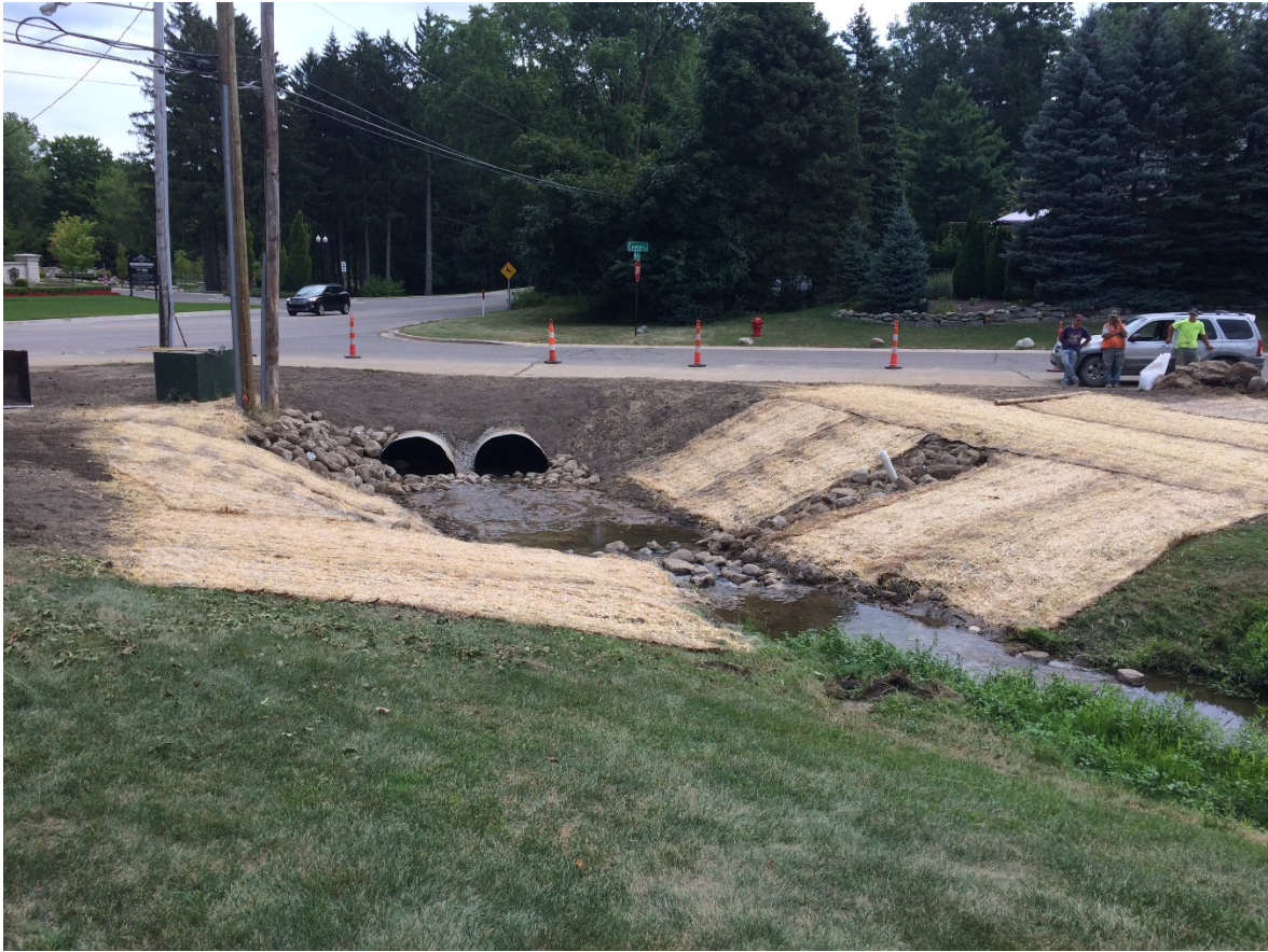
Thornton Creek culvert crossing at 9 Mile and Center Street – start of restoration.
