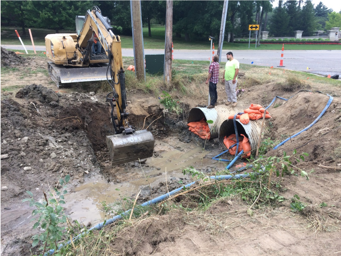
Thornton Creek culvert crossing at 9 Mile and Center Street - clearing and grading.
