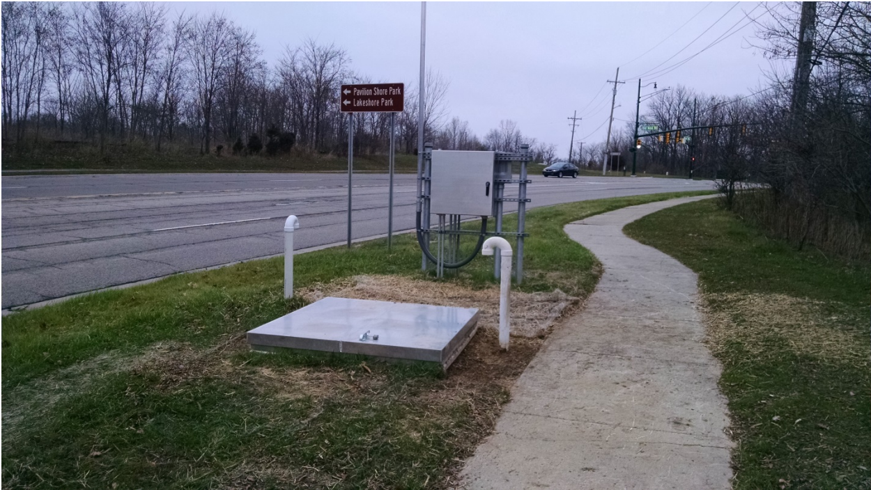
Close-up of PRV station
