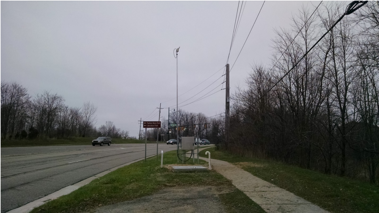
Overall of PRV station – east-side of Novi Road, south of Old Novi Road
