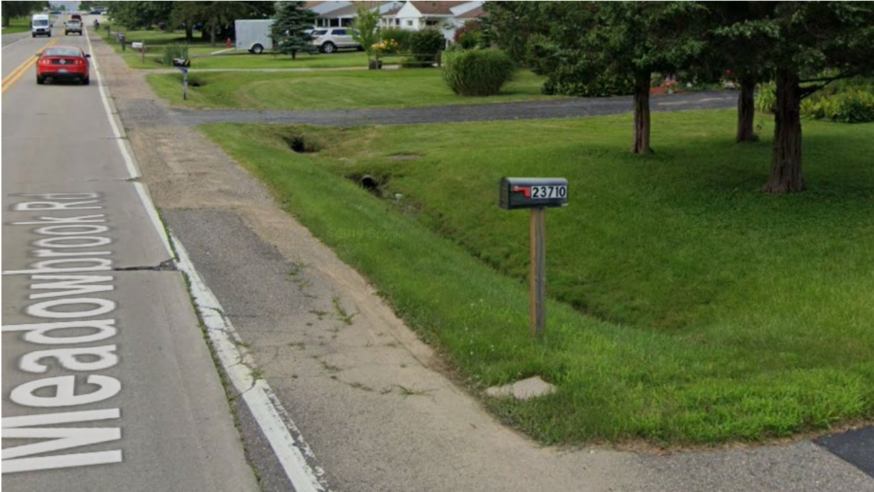
Example of an Open Ditch on Meadowbrook Rd
