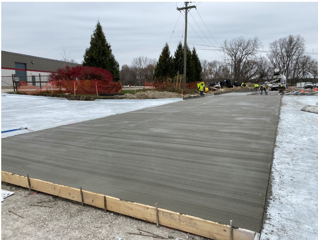
Pouring the southbound lanes of Crescent Boulevard and driveway for General Filters.
