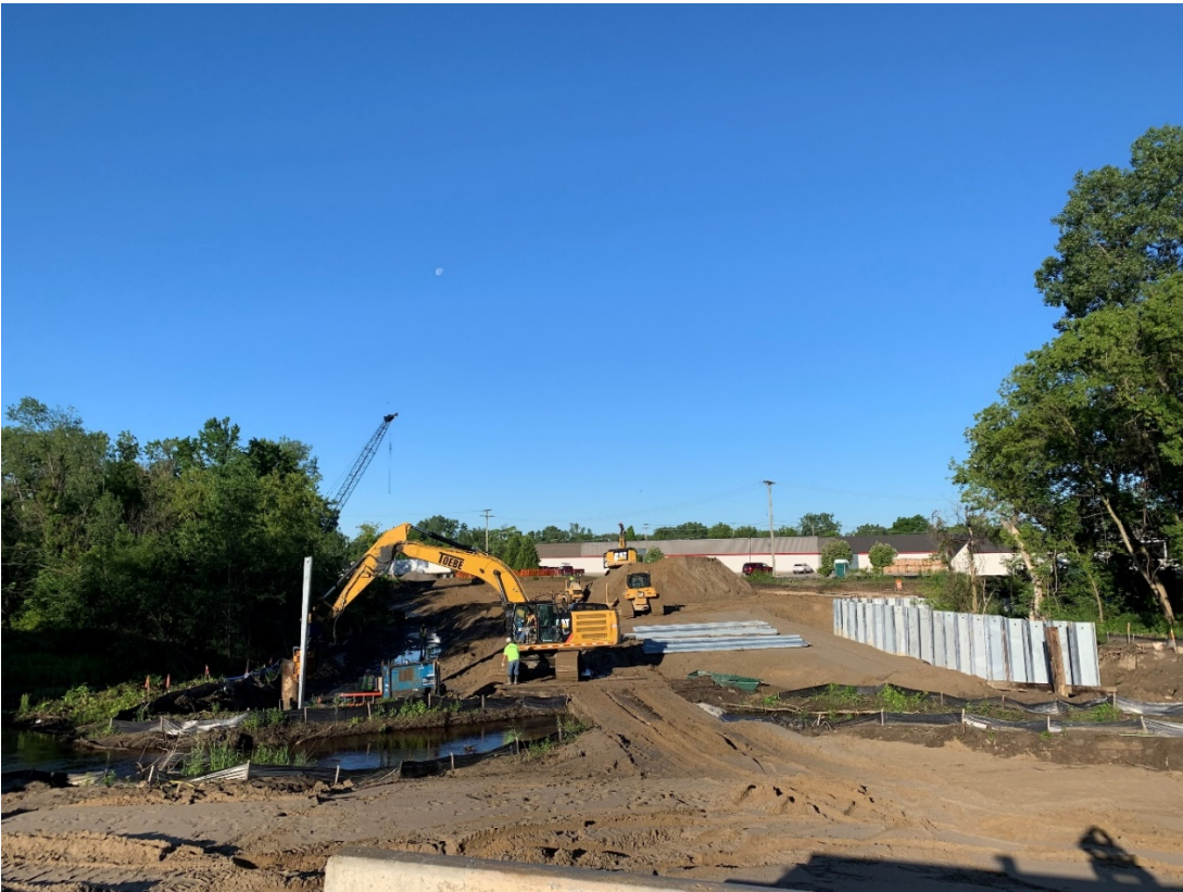
Installing sheeting and forms for the walls on each side of the Middle Rouge River.
