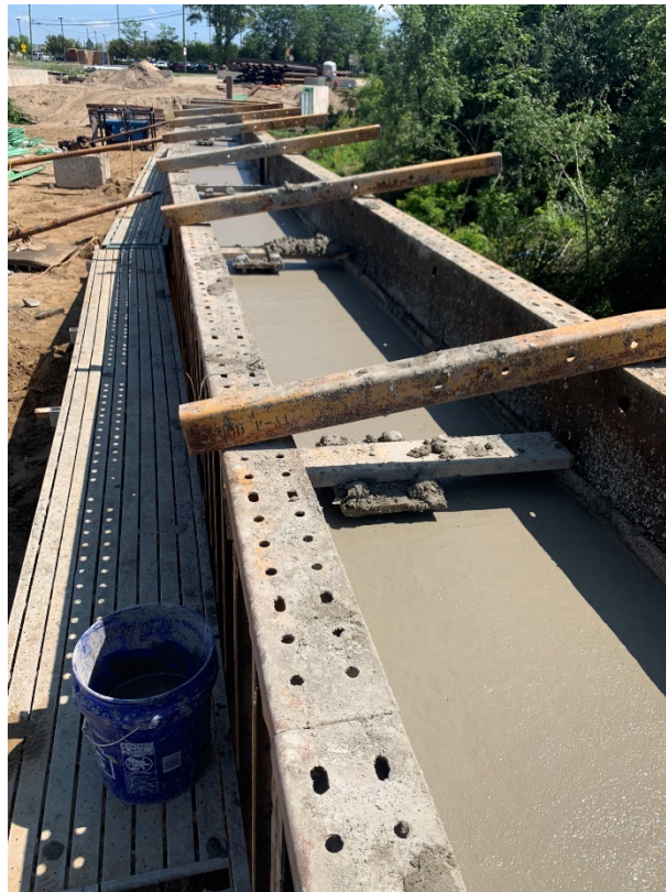
Wall forms and poured concrete for Crescent Boulevard, SW corner of river.
