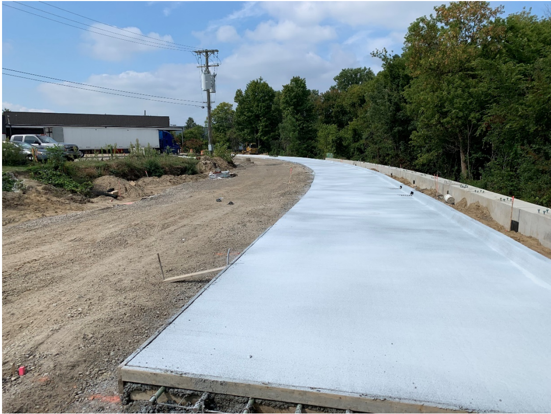
Completed concrete pour of the north ½ of the Industrial Spur (Lambert Drive).
