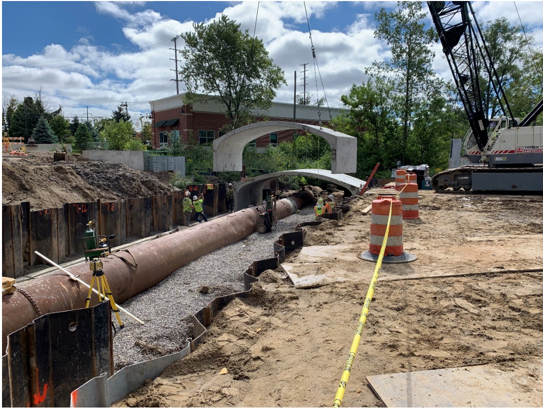
Installing the new modified box culvert over top the Middle Rouge River by-pass.
