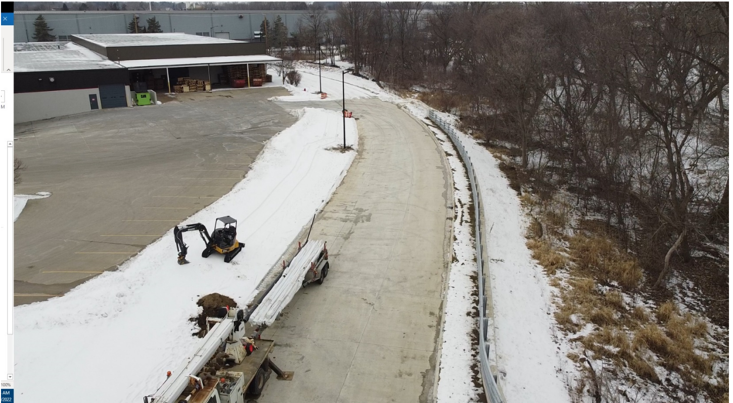
DTE Streetlighting Division installing new LED streetlights along Industrial Spur (Lambert Drive).
