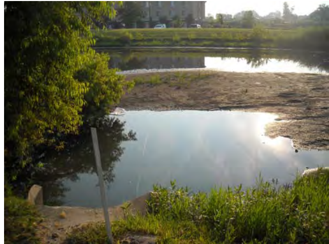
Sediment Accumulation at Basin #2
