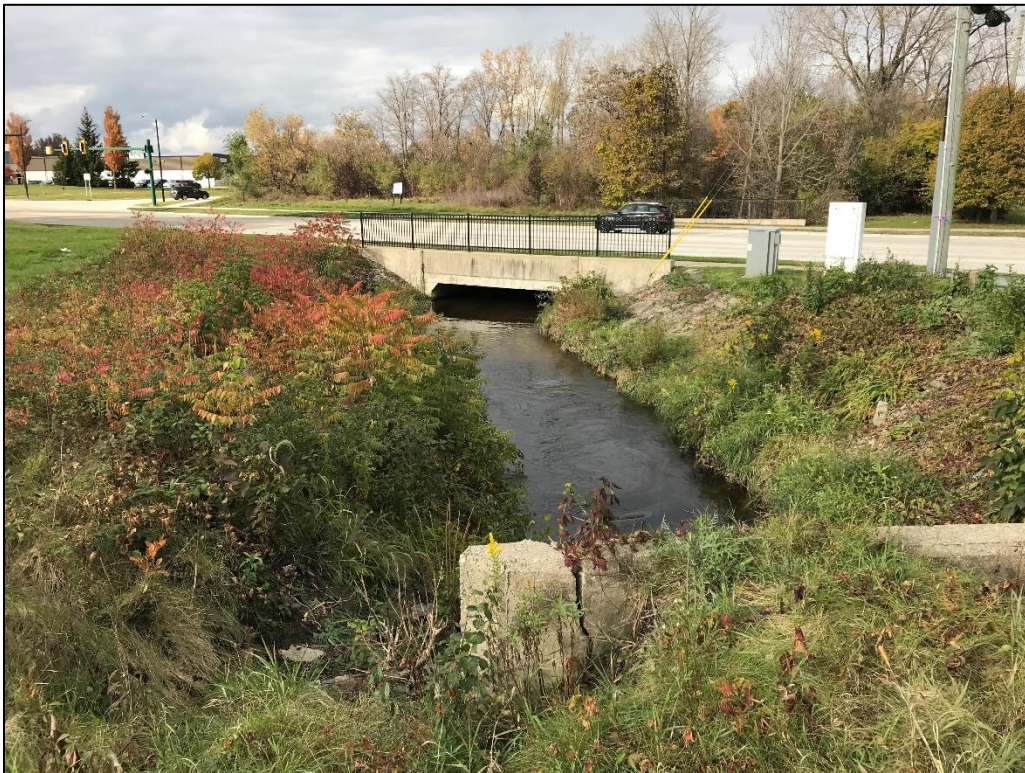
Photo 2: View of the regulated wetland area, facing northwest. Note the crack in the concrete headwall in the foreground.
