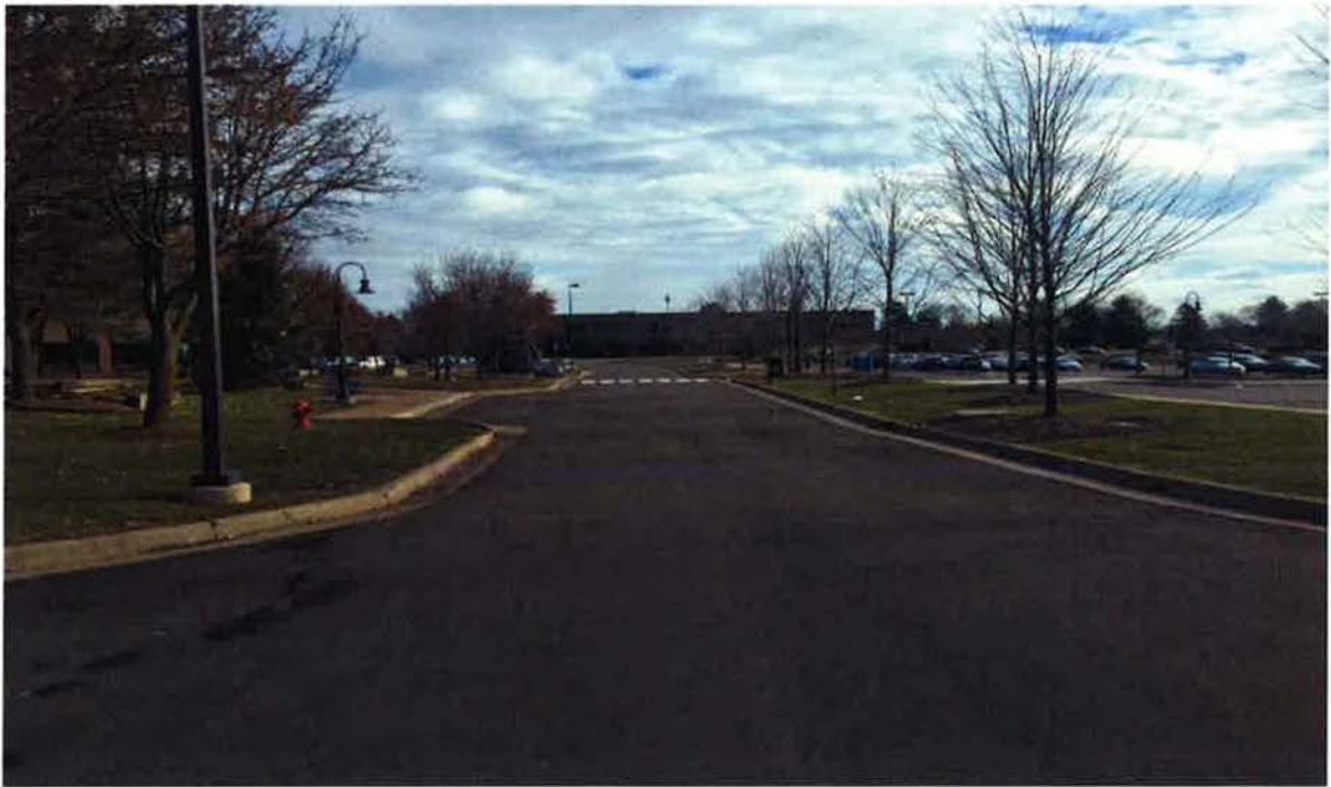
New asphalt pavement on Novi Way at main entrance to Civic Center
