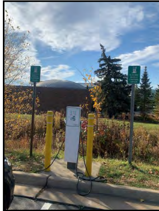
Figure D15: electric vehicle charging stations at the Novi Public Library; see subsection 5.2.15 for details on EV charging stations
