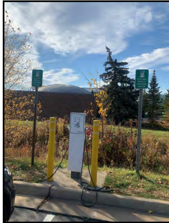
Figure D15: electric vehicle charging stations at the Novi Public Library; see subsection 5.2.15 for details on EV charging stations
