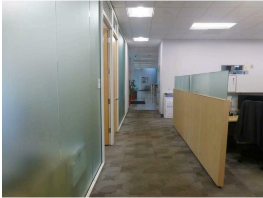
2nd View Office LED Lighting
