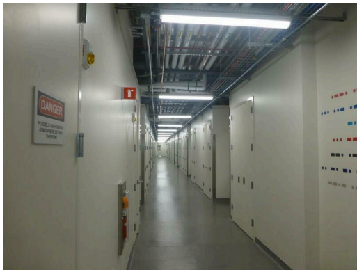
Corridor LED Lighting
