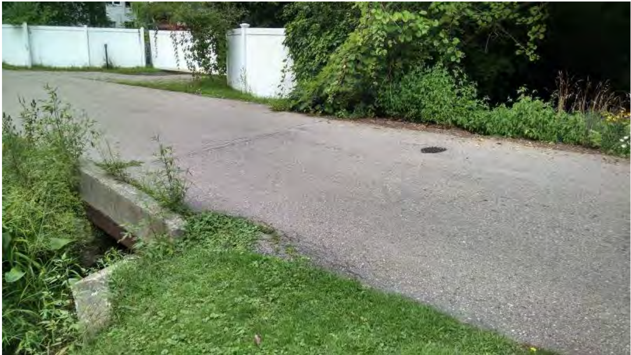
Sink Hole Recently Observed
