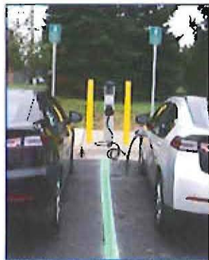
Electric vehicles charging station located at the Novi Police Headquarters.
