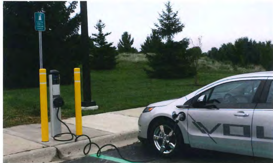
PEV Charging Station and Space (Novi Police Station)
