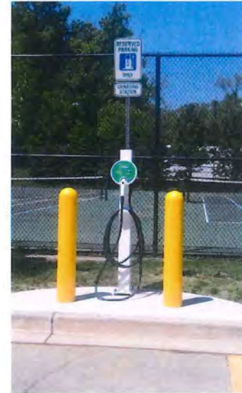
PEV Charging Station and Space (Auburn Hills, MI)
