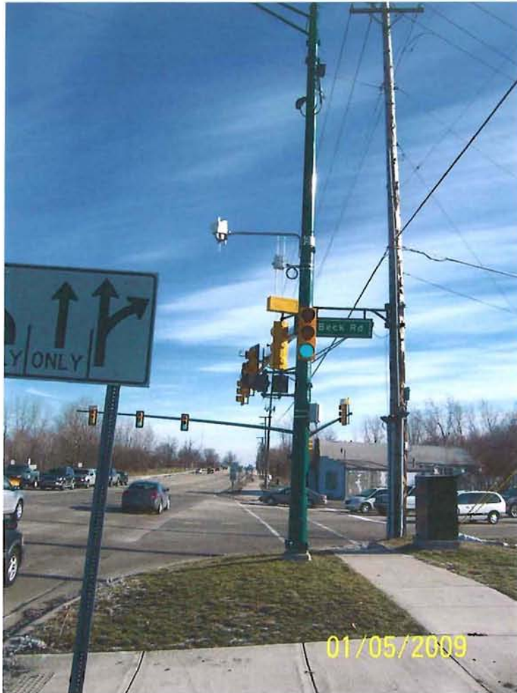
Existing wood pole on SW corner to be used for street lighting
